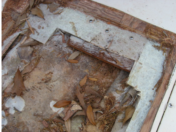
Figure 5 Close up of cleat under deck with screws to hold while epoxy cures
